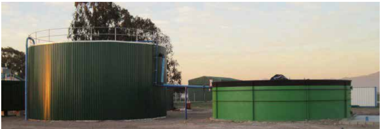
Figure 2.8: Zandam Farm plant (Anaergia)
